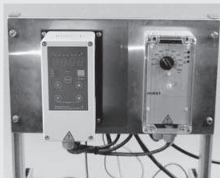
Heat control system for THTMD
