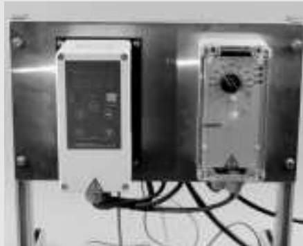
Heat control system for THTMD
